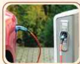
Electric Vehicle Charging Point
