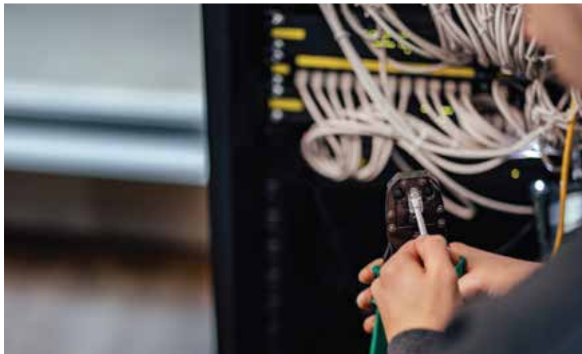
Wiring Copper Electrical Wiring throughout in concealed conduit(ISI Marked)
