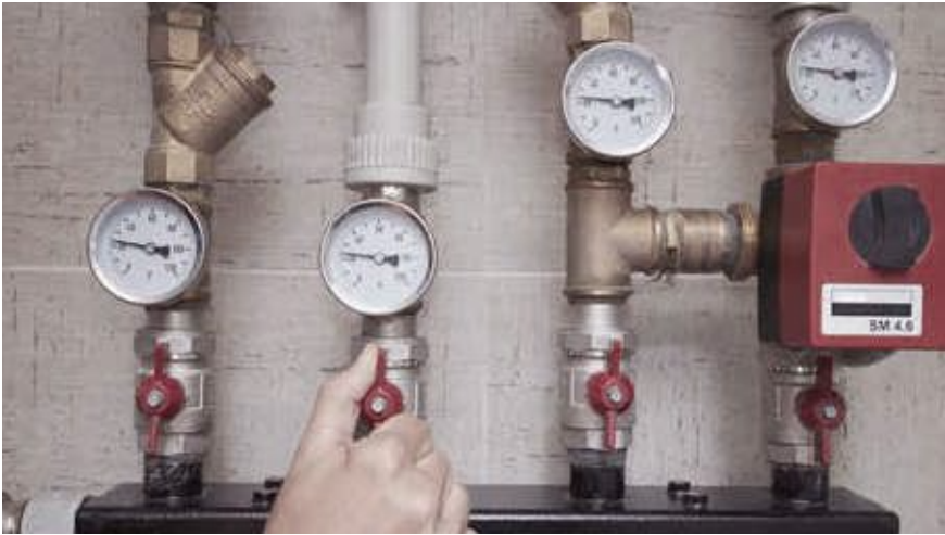
Smart Meter for Water and Electricity
